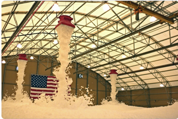
Fire suppression systems
